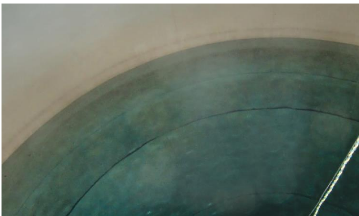
Figure 3c. Image of tank after operation of the mixer. Despite sub-freezing temperatures, the tank was rendered ice-free after a week of mixer operation.
