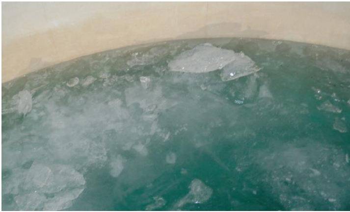
Figure 3a. Ice conditions inside the tank prior to turning on the mixer. Note the damaged coatings above the water line.
